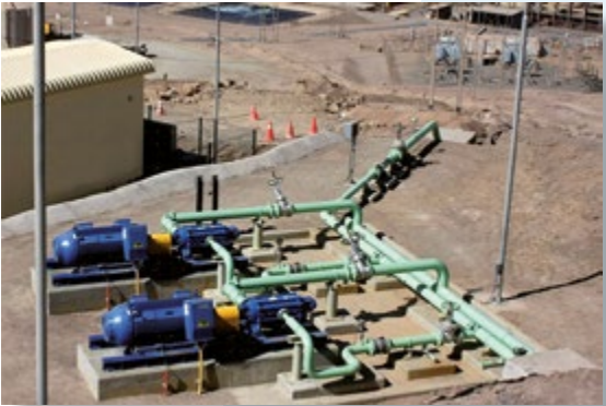
Water Booster Pumping Station Horizontal Multistage Pumps HR 150™-6E
